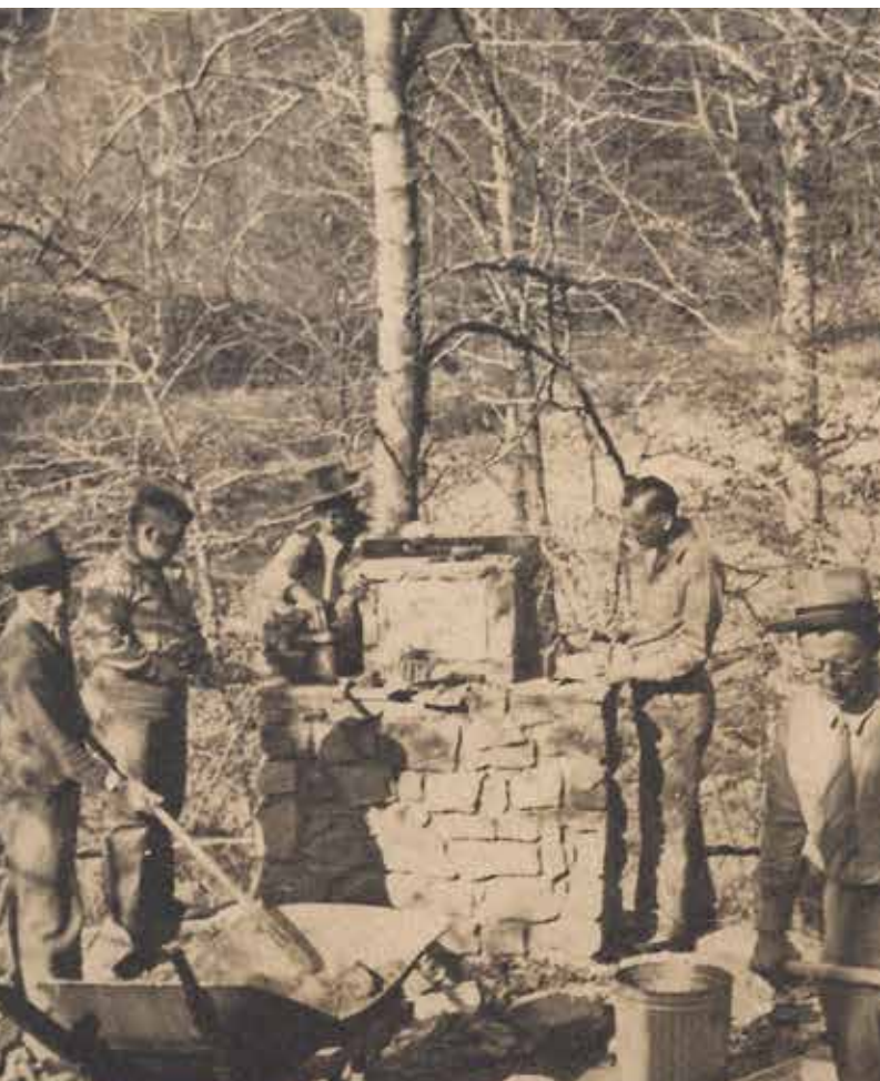
Banks Newman (second from right) works with Scouters to construct the Tom Holder Memorial Chapel at Camp Lasater in 1945. Courtesy of Raven Knob Boy Scout Museum, Old Hickory Council, BSA
